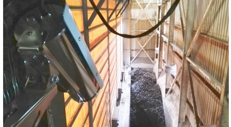
FireTIR monitoring in cement factory
